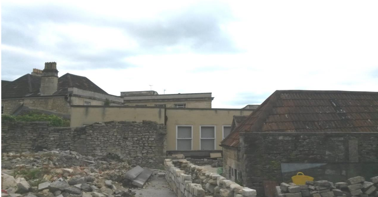
Photo from rear of No. 24 Silver Street that would face new roof addition and stairway
